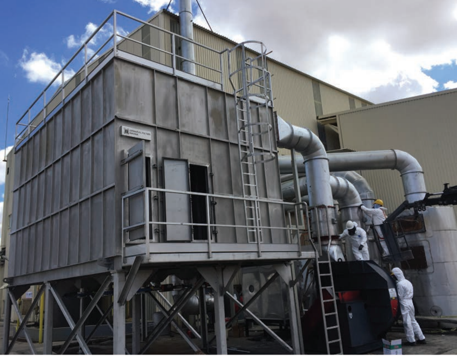
Altın Madeni Gaz Filtreleme Sistemi Gold Mine Gas Filtration System
